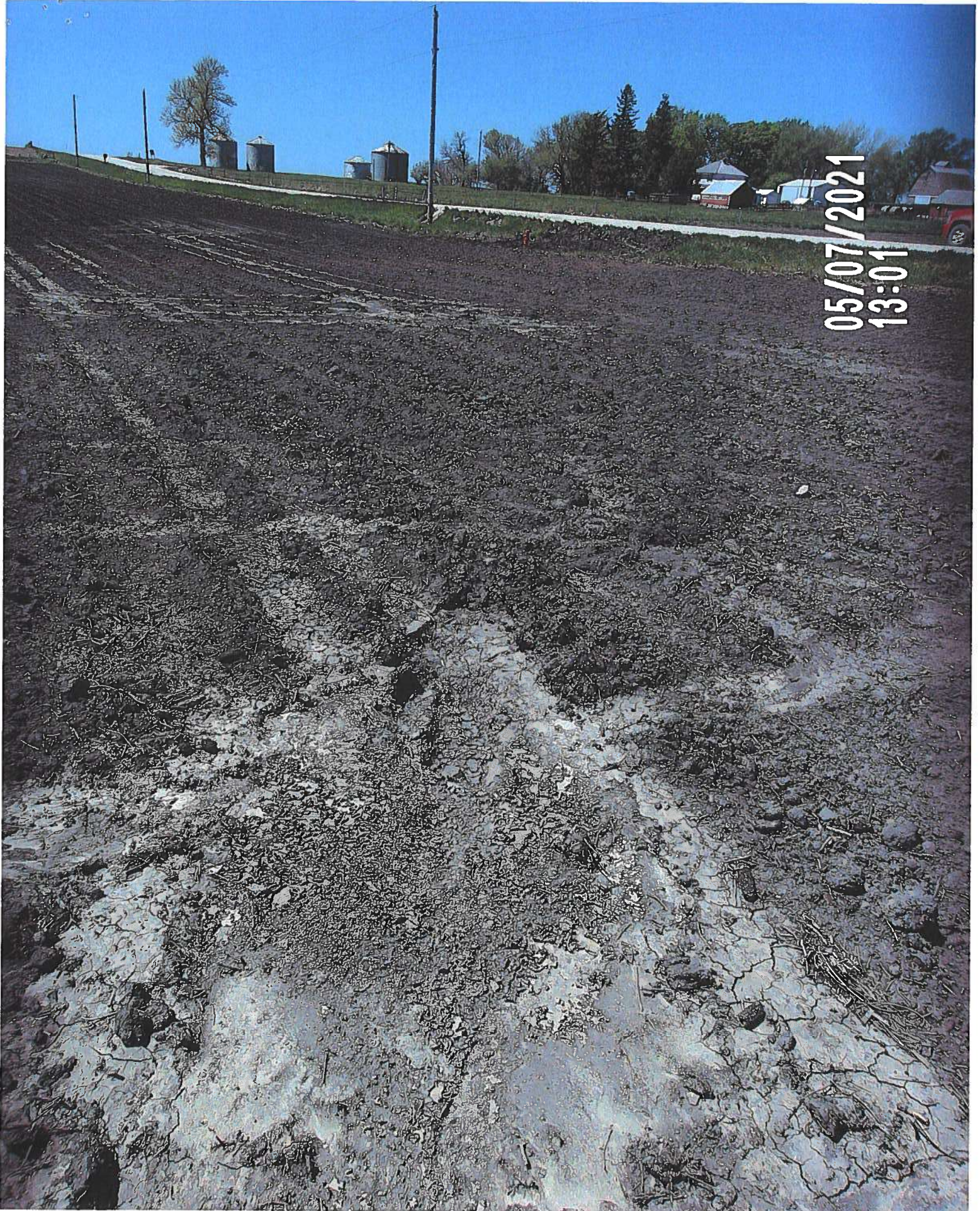
LOOKING UPSTREAM ON S. SIDE OF 110TH ST. @ WATER EROSION.
